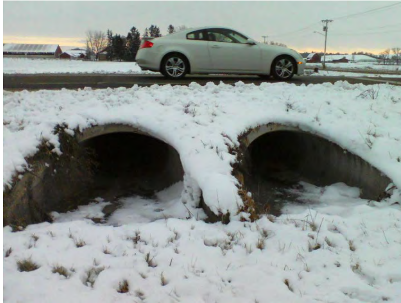
Figure 6-4. Twin 30 inch by 45 inch culverts under Lacy Road immediately east of Seminole Highway.
