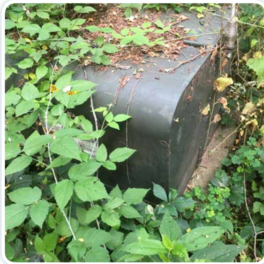
Figure 23. MG&E electrical box in the North Park Addition
